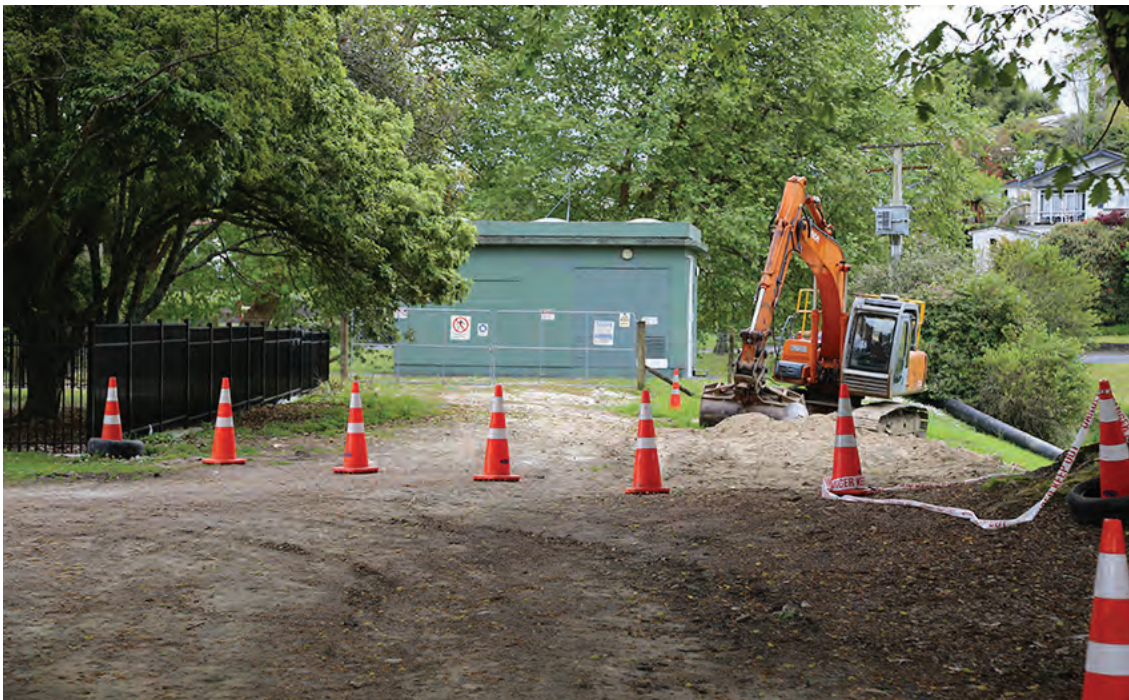
MAIN PUMP STATION TE KUITI
